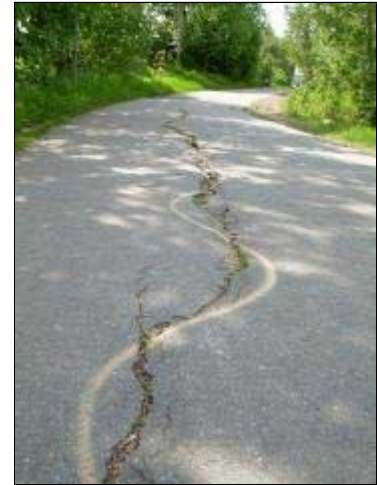
A long crack on the Tony Knowles Coastal Trail west of Lyn Ary Park is an example of repairs that don't get done in city parks and trails. ( BROOKE BLESSING, Municipality of Anchorage )
